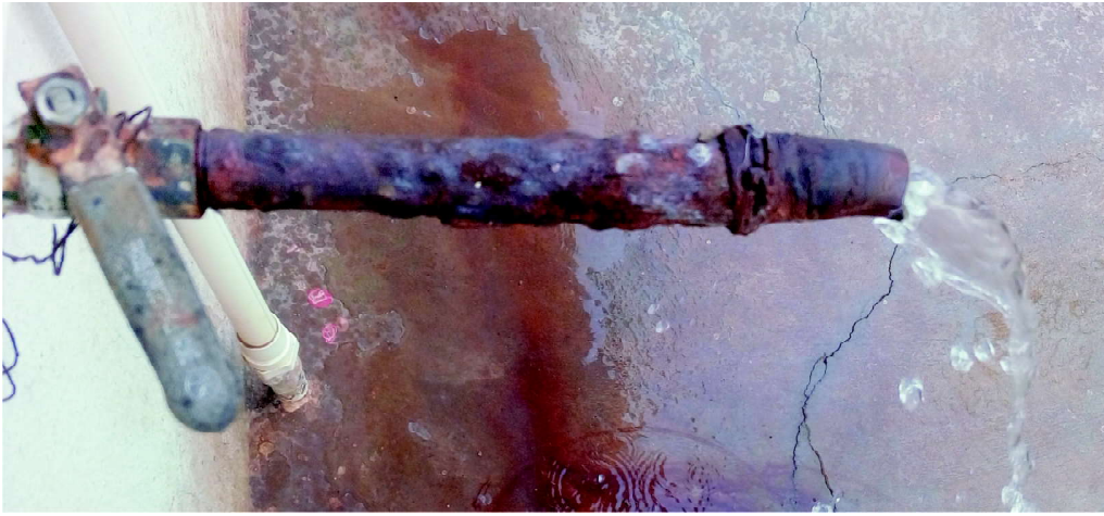
Fig. 8.4: Process of rusting on iron tap.
